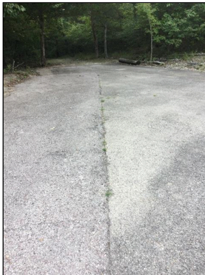
1.5 Instance of crack, weathered surface
