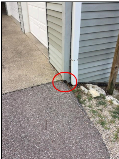
1.0 Instance of damage
