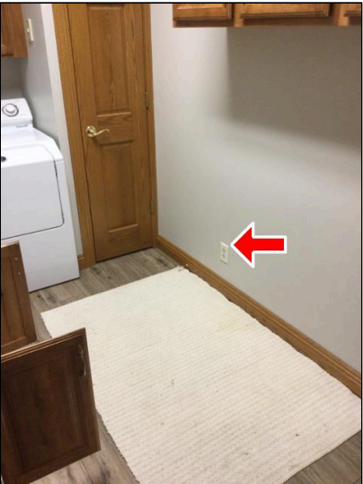
7.8 Instance of outlet lacking GFCI protection - laundry
