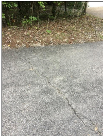
1.5 Instance of crack, weathered surface
