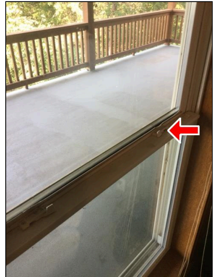
3.9 Instance of damage, hard to operate - lower level living room
