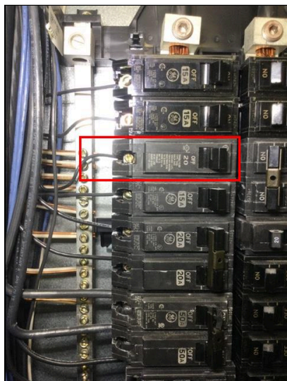
7.4 Over amp breaker
