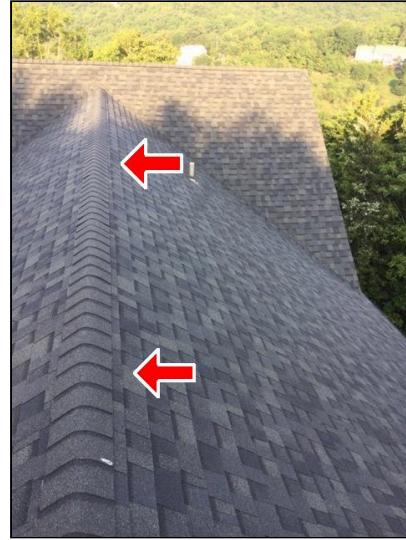
8.3 Ridge vent not installed
