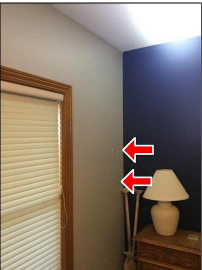
3.2 Instance of nail pops (behind painted wallpaper) - master bedroom
