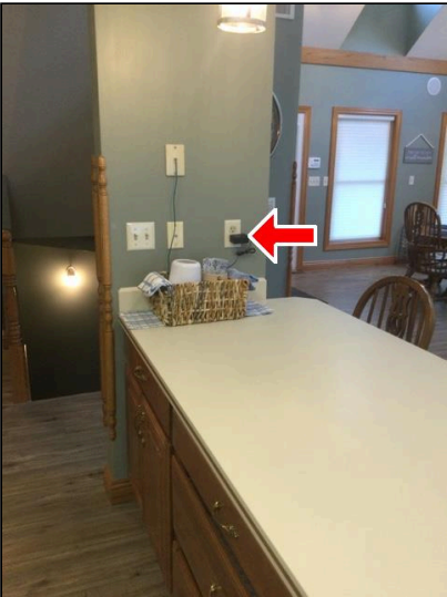
7.8 Instance of outlet lacking GFCI protection - kitchen
