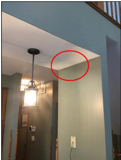
3.2 Instance of repair attempt - kitchen
