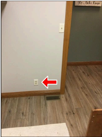
7.8 Instance of outlet lacking GFCI protection - laundry
