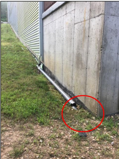
1.4 Instance of maintenance/ improvement needed
