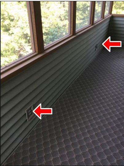
7.8 Instance of outlet lacking GFCI protection - rear covered deck
