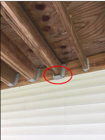
1.3 Improper joist hanger
