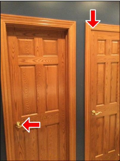
3.8 Instance of maintenance/ adjustments needed - master bath (closet door did not latch, linen door rubbed jam)
