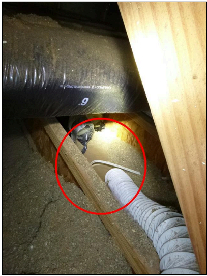
8.3 Bath exhaust vent termination
