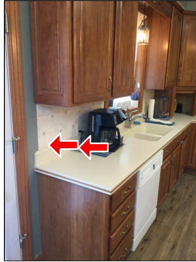
3.4 Instance of silicone maintenance needed
