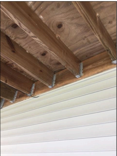
1.3 Joist hangers lacked some nails where required
