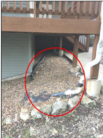
1.4 Instance of maintenance/ improvement needed
