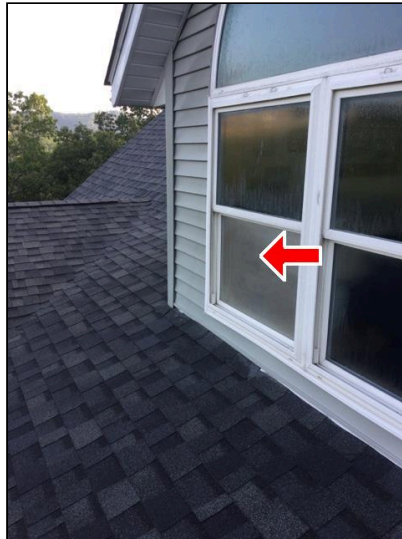
3.9 Instance of moisture/cloudy panes
