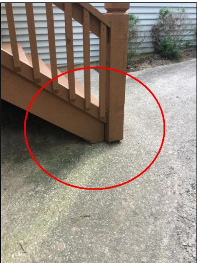
1.3 Instance of decay/ deterioration/damage, weak guard
