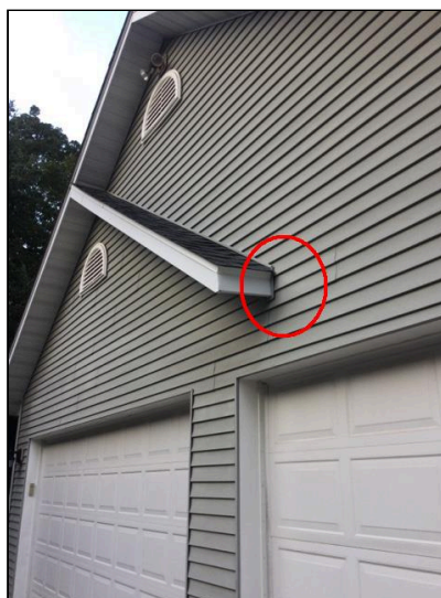
2.2 Instance of inadequate flashings
