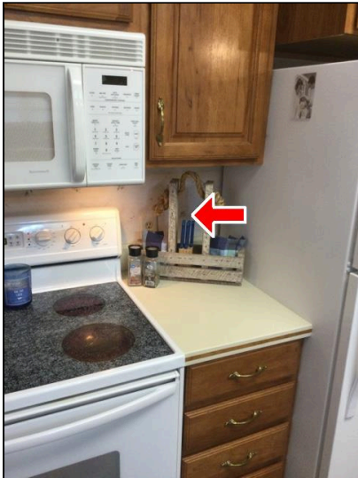
7.8 Instance of outlet lacking GFCI protection - kitchen
