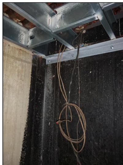
7.5 Instance of sub-standard install - under patio room (exposed wires)
