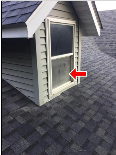
3.9 Instance of moisture/cloudy panes
