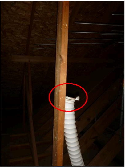
8.3 Bath exhaust vent termination
