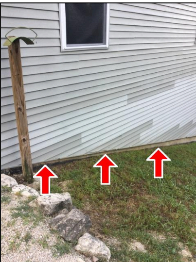
1.0 Instance of damage
