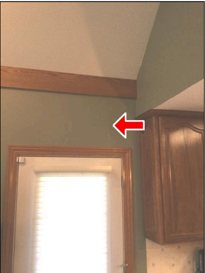
3.2 Instance of cracks/separations - living room/kitchen
