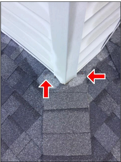
2.1 Instance of exposed nail
