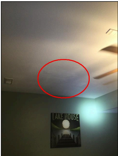
3.2 Instance of repair attempt - lower level
