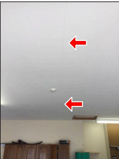
3.2 Instance of cracks/separations - garage
