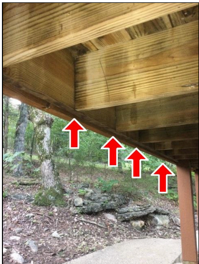
1.3 Instance of joist hangers not installed
