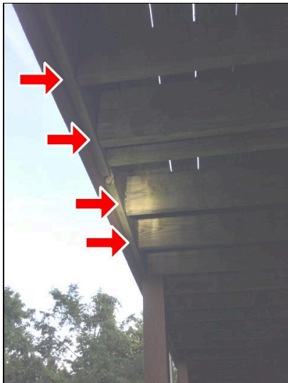
1.3 Instance of joist hangers not installed, withdrawn connections
