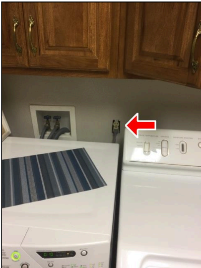
7.7 Instance of cover not installed - utility room
