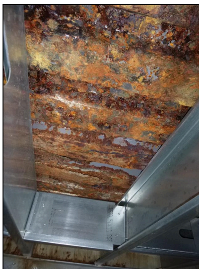
4.6 Rusty metal deck underneath the concrete
