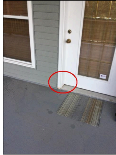
1.0 Instance of damage, repair needed
