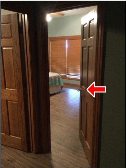
3.8 Instance of maintenance/ adjustments needed - lower bedroom
