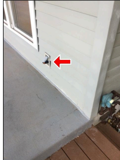
7.8 GFCI did not trip - lower rear exterior
