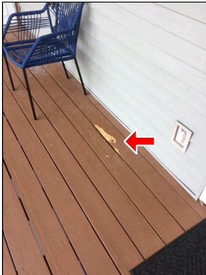
1.3 Finish in need of improvement
