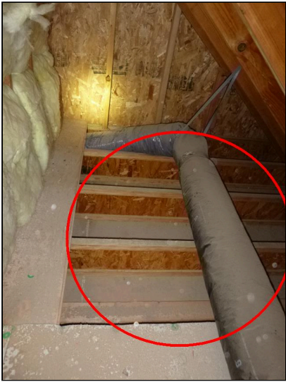
8.2 Very little insulation above master bathroom area
