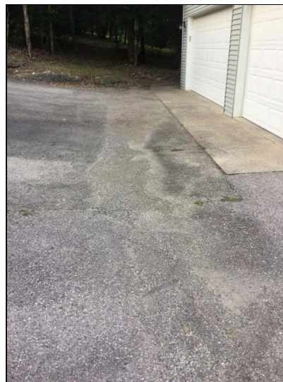
1.5 Drainage in need of improvement
