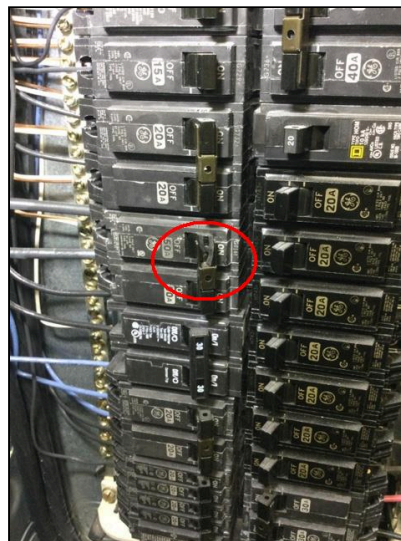
7.4 Damaged trip handle
