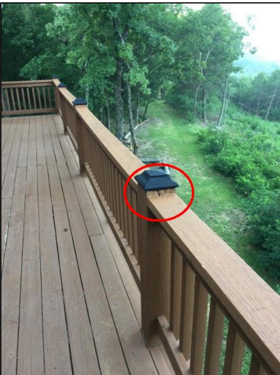
1.3 Instance of decay/deterioration/damage
