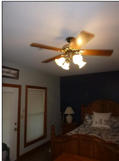
7.6 Instance of noisy fan - master bedroom
