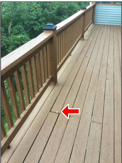
1.3 Instance of loose board
