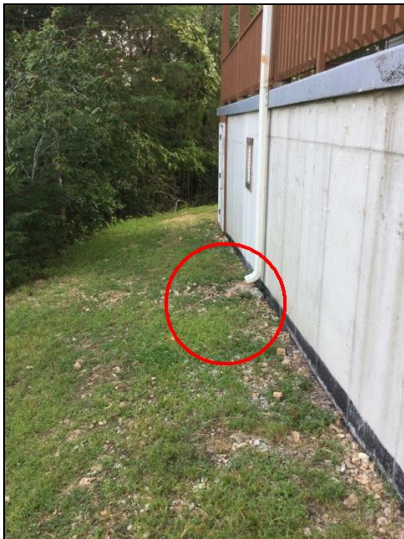
1.4 Instance of maintenance/ improvement needed
