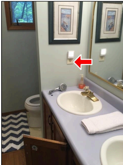
7.7 Instance of ungrounded 3-prong outlets - lower bathroom
