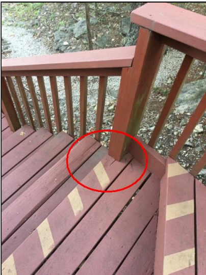
1.3 Instance of decay/deterioration/damage
