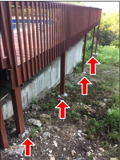
1.3 Instance of concrete poured around posts, susceptible to moisture damage/decay
