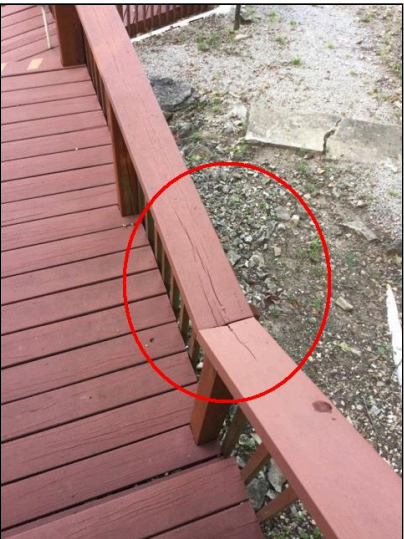
1.3 Instance of decay/ deterioration/damage
