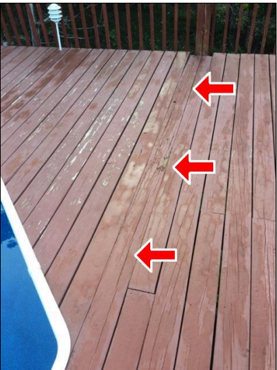
1.3 Instance of decay/ deterioration/damage
