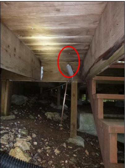
7.5 Instance of sub-standard install - under deck shelter/ pool room
