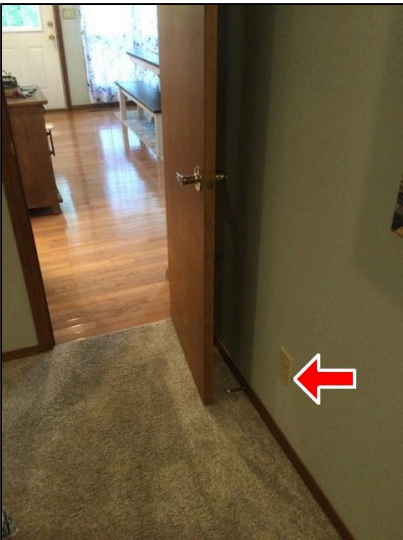
7.7 Instance of loose outlet - main level bedroom
