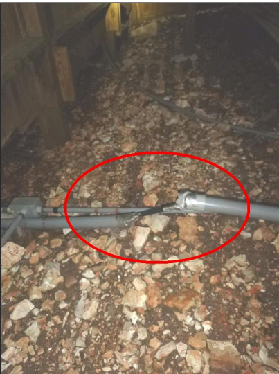
7.5 Instance of sub-standard install - under deck (damaged conduit)
