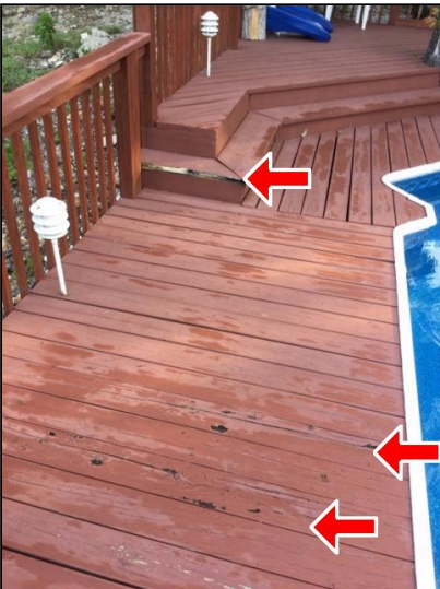
1.3 Instance of decay/ deterioration/damage
