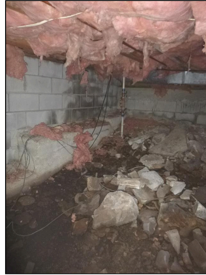
4.3 Moisture in crawlspace
