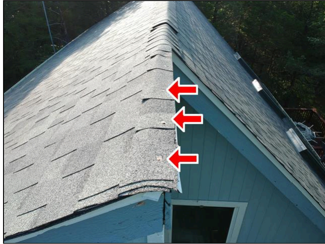
2.1 Instance of sealant needed at fasteners
