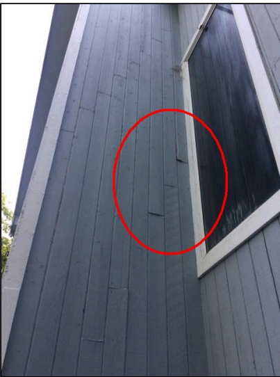
1.0 Instance of repairs needed
