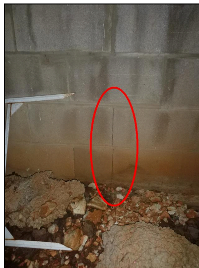
4.2 Instance of tuck pointing needed
