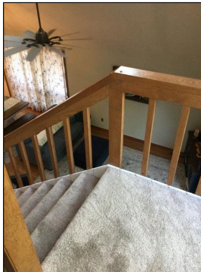
3.6 Spindle spacing in need of improvement, graspable handrailing not installed
