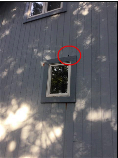
1.0 Instance of repairs needed
