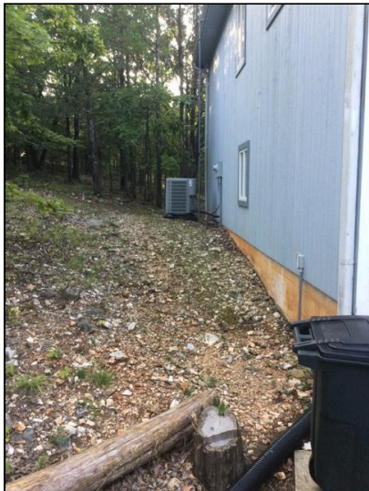
1.4 Instance of maintenance/ improvement needed
