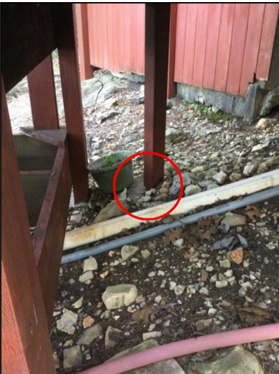
1.3 Gap between post and footing
