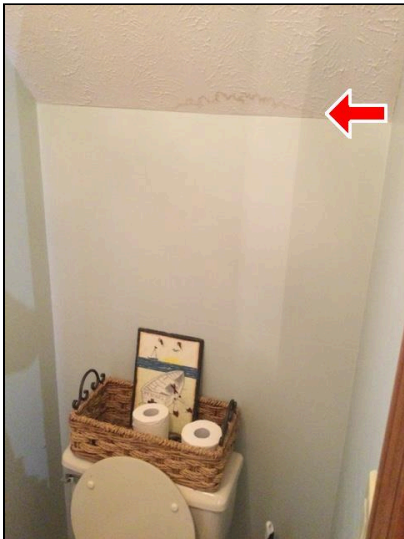
3.2 Instance of stains - upper bathroom
