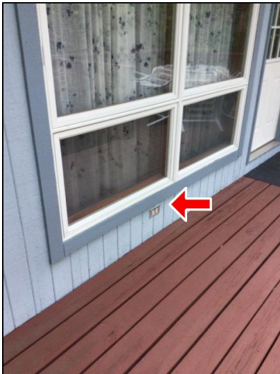
7.7 Instance of damaged cover - deck
