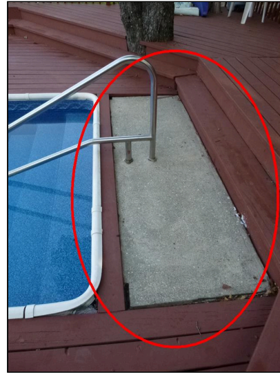
14.24 Potential trip hazards
