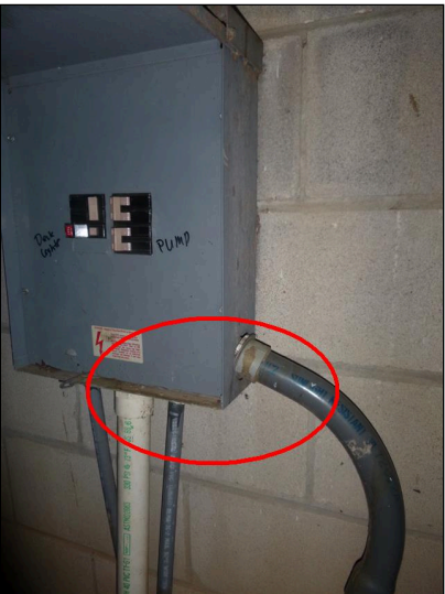
7.5 Instance of sub-standard install - panel under deck (damaged conduit connections)
