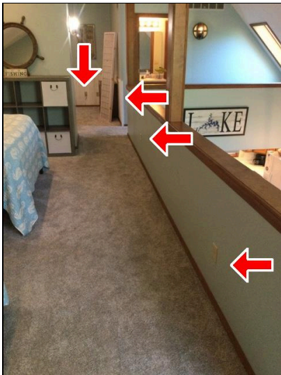
7.7 Instance of ungrounded 3-prong outlets - upper level
