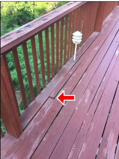
1.3 Instance of decay/ deterioration/damage
