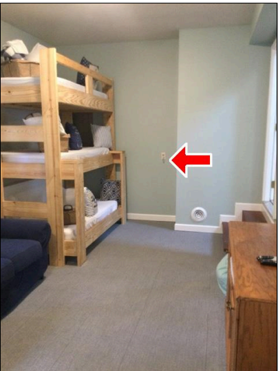
7.7 Instance of ungrounded 3-prong outlets - lower bedroom
