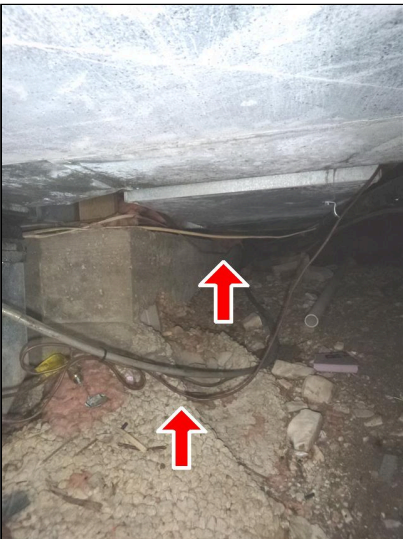
7.5 Instance of sub-standard install - crawlspace (inadequately secured)
