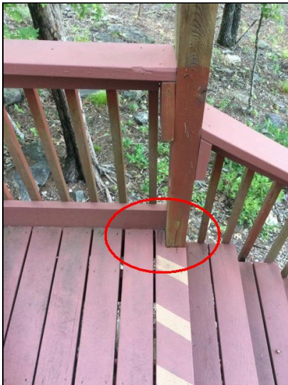
1.3 Instance of decay/ deterioration/damage
