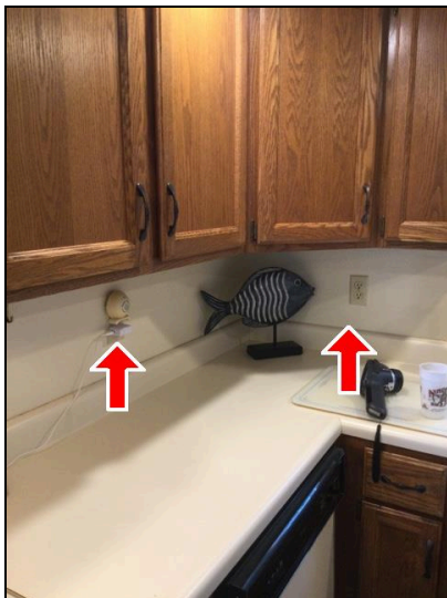
7.8 Instance of outlet lacking GFCI protection - kitchen
