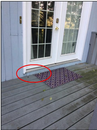
1.0 Instance of decay/deterioration/damage
