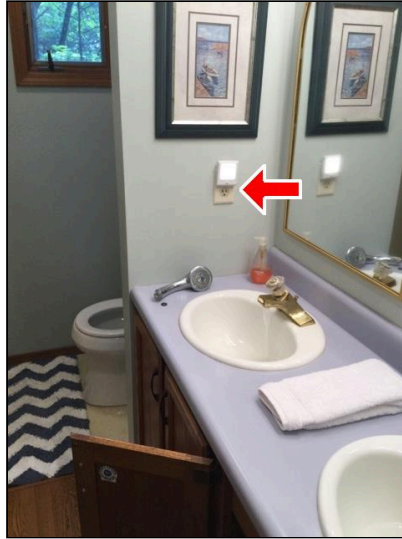
7.8 Instance of outlet lacking GFCI protection - main level bathroom
