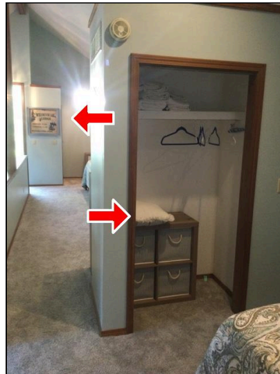
3.8 Instance of doors not installed
