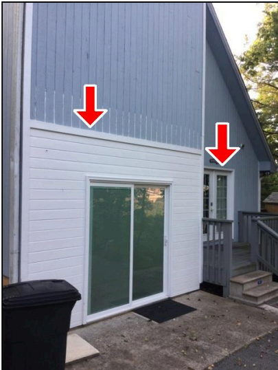
1.0 Instance of flashings not observed
