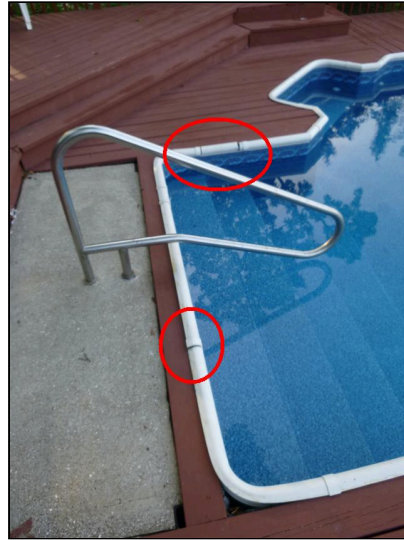
14.2 Gaps, inadequately secured
