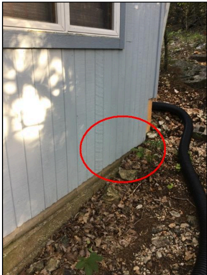
1.0 Instance of decay/ deterioration/damage
