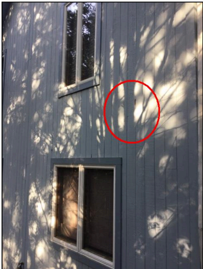
1.0 Instance of repairs needed
