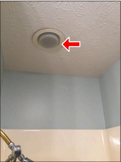
7.6 Instance of lighting that did not respond - bathroom
