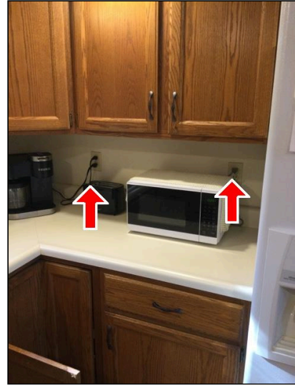
7.8 Instance of outlet lacking GFCI protection - kitchen
