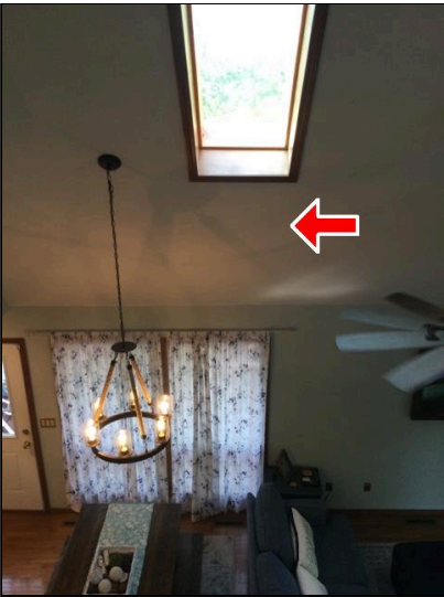
3.2 Instance of stains - skylight ceiling
