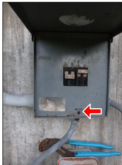
7.3 Screw not installed
