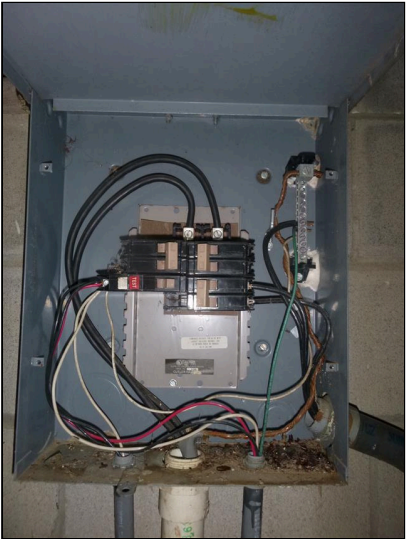
Exterior panelboard (under deck)
