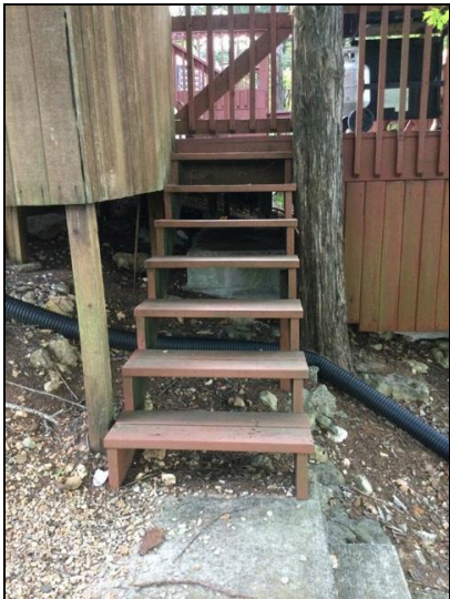
1.3 Inconsistent tread height, guard railing not installed
