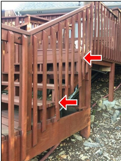
1.3 Loose railing components
