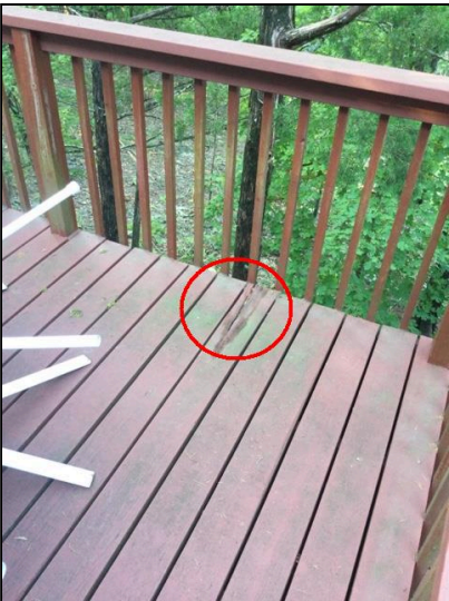
1.3 Instance of decay/deterioration/damage
