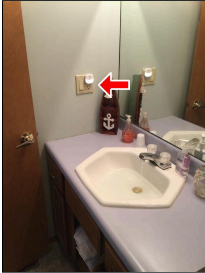
7.8 Instance of outlet lacking GFCI protection - upper bathroom
