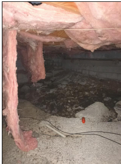
4.8 Instance of damaged/displaced insulation
