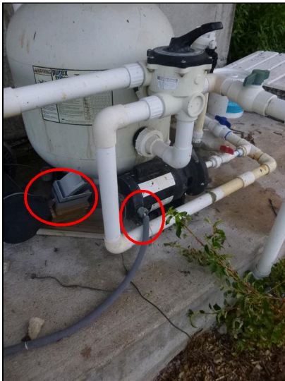
7.5 Instance of sub-standard install - pool pump area (damaged conduit)
