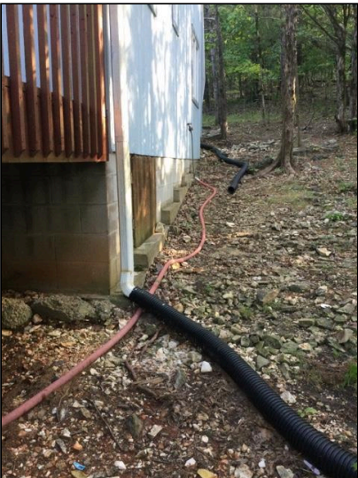
1.4 Instance of maintenance/ improvement needed
