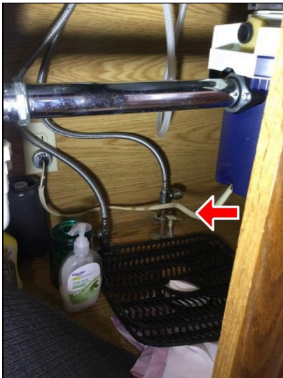
7.5 Instance of sub-standard install - kitchen disposal (romex used as appliance cord)
