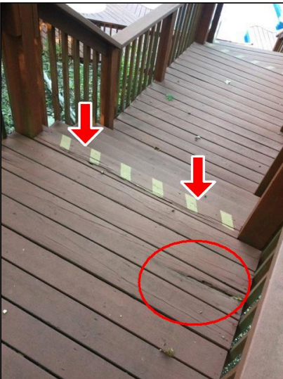
1.3 Instance of decay/ deterioration/damage
