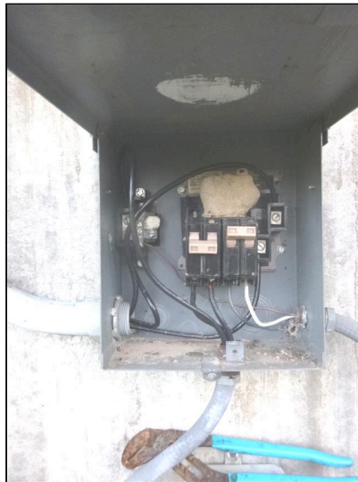
7.3 3 wires in feeder bundle (at pool pump)
