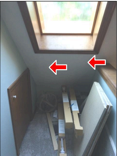
3.2 Instance of stains - skylight ceiling
