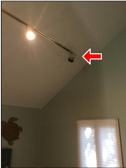
7.6 Instance of lighting that did not respond - upper level
