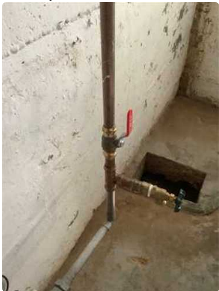
Main water shut off front wall
